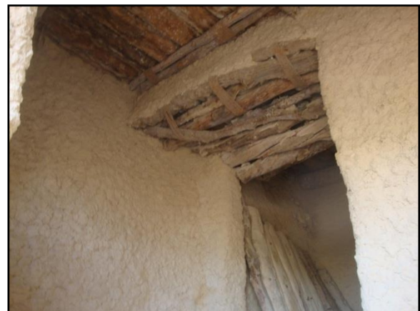
Figure 8. The use of wood in joining the walls and roofing of one of the old houses in Shali Castle built from Al-Kurshef
