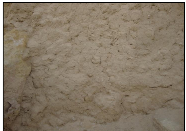
Figure 30. Salt fluorescence on the surface of the mortar due to the saline nature of Al-Kurshef - Shali Castle
