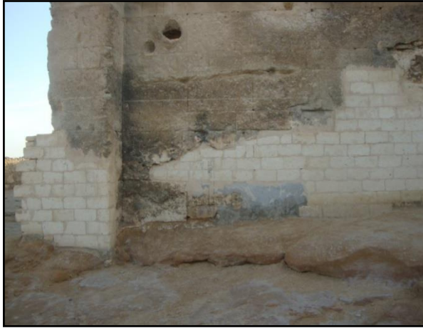
Figure 26. One of the completion of the walls of the Temple of Oracle, as a result of the weakness and erosion of the saline limestone
