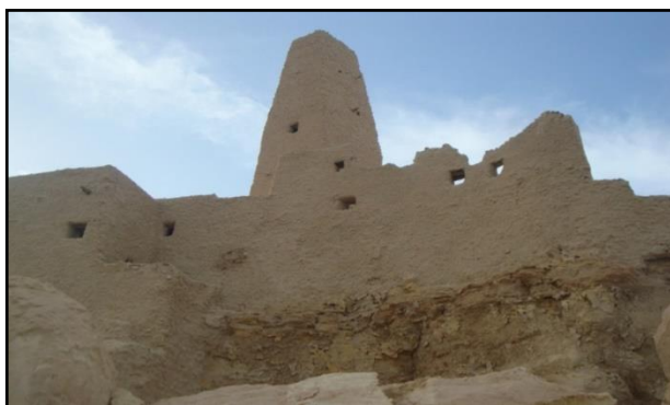
Figure 28. Al-Kurshef is damaged and eroded at the bottom of one of the walls of the historic Shali castle, which exposes it to partial or complete collapse
