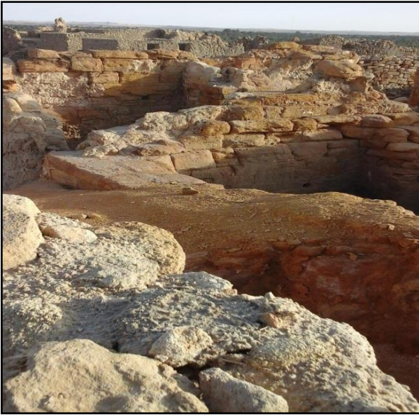
Figure 21. The crumbling and degradation of the saline limestone at the Temple of Oracle in Siwa
