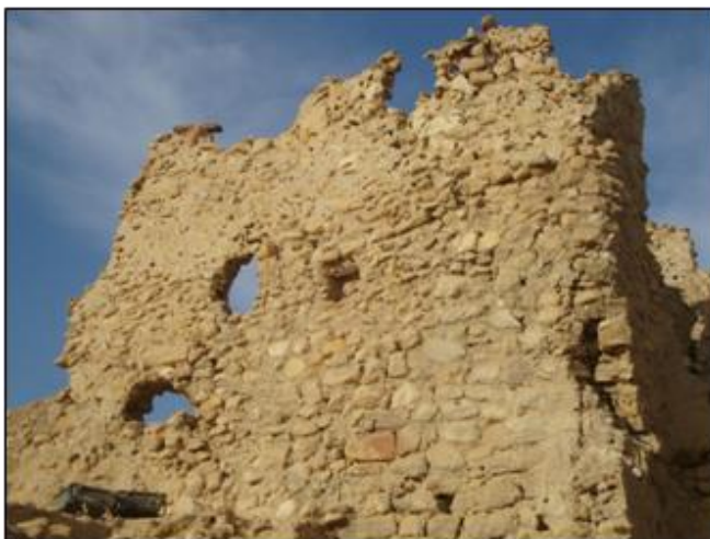
Figure 7. One of the walls in Shali Castle, which was built from Al-Kurshef, and it becomes clear that there are deep cracks and separation in the walls.
