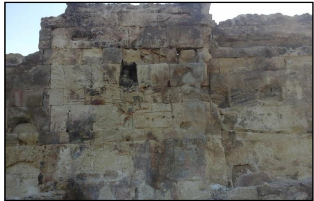
Figure 24. Saline limestone eroded and cracks spread in one of the walls - the Oracle temple
