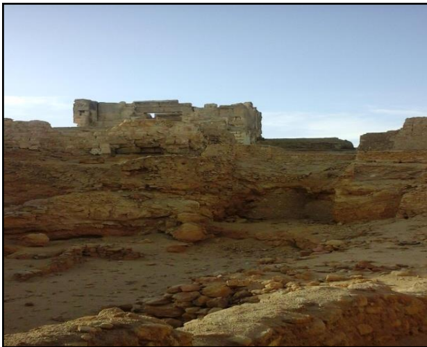
Figure 27. The Aghurmi rock, on which the Temple of Oracle is built, is threatened with collapse at any time, threatening the security and safety of the temple
