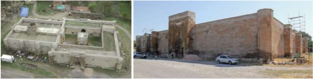
Figure 17. Ağzıkara Han, before (Eravşar, 2017; photo I. Dıvarcı) and during restoration (photo: I. Simon, 2015).
