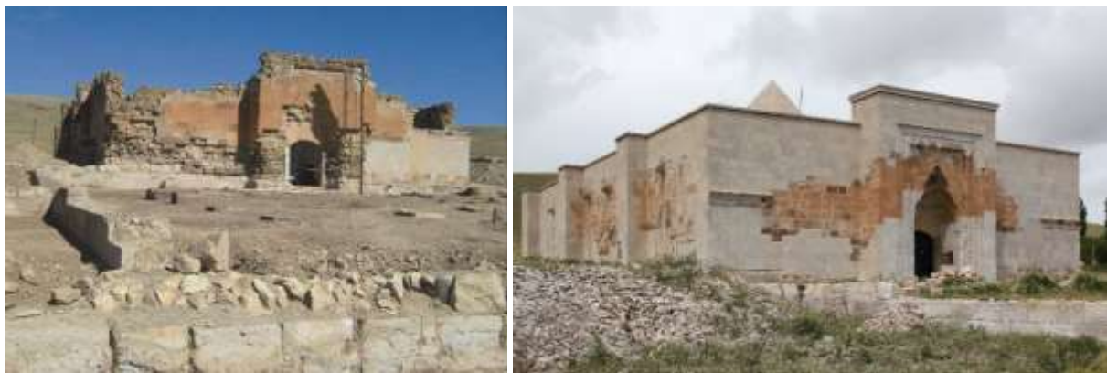
Figure 16. Alay Han, before (Eroşar, 2017; photo I. Dıvarcı) and after (photo I. Simon, 2016) restoration.
